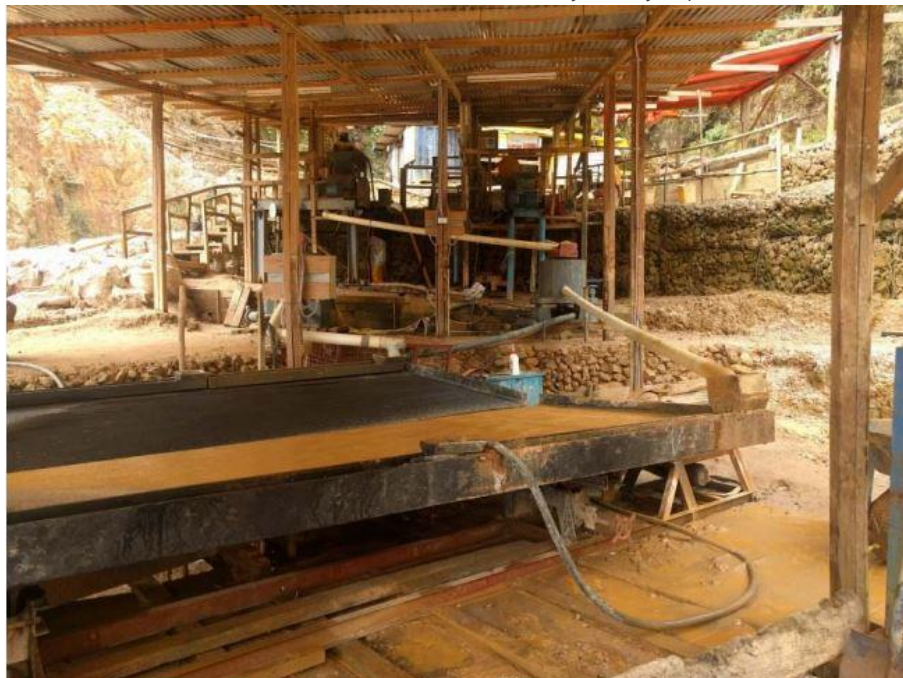
Figure 46: 2016 HGV Mine processing plant upgrade: hammer mills, centrifugal concentrators and shaking tables. (Source: ASX:CGN 7 June 2016)
