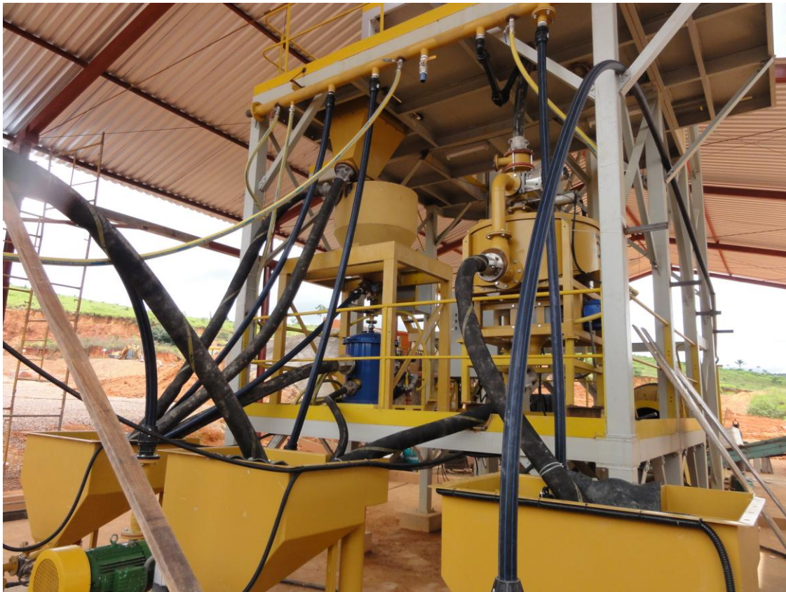
Gekko Gravity Concentrating Plant at Sao Chico
